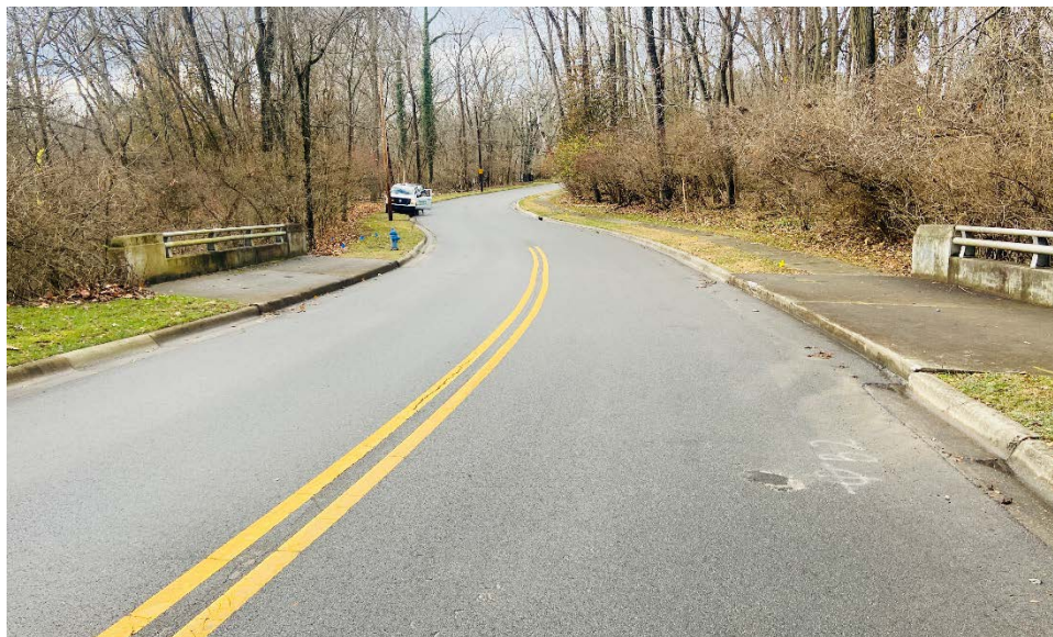
Photograph 1: Pavement Condition of W Selby Blvd
