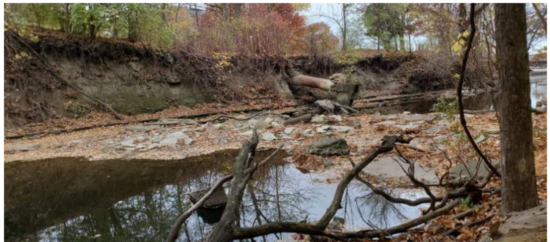
Figure 3: West Bank Erosion/Outfall Structure Failure.
